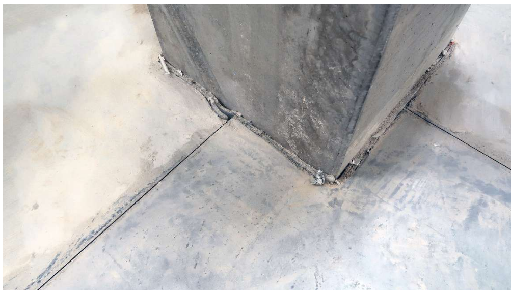
Figure 5. Opening of the steel expansion joint at a column line after shrinkage deformation
